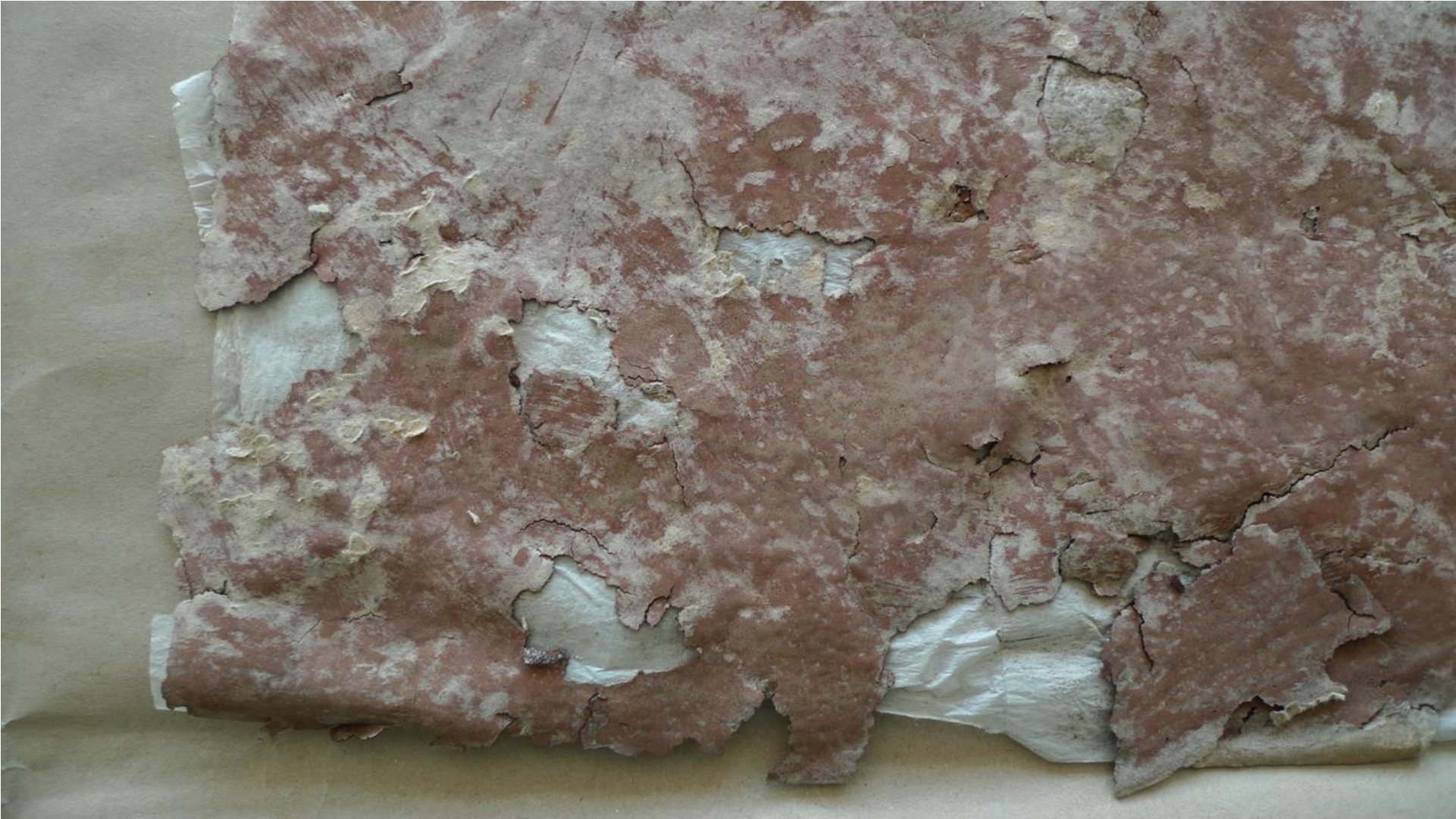
Lower areas of wallpapers can be significantly more damaged and paper become completely soiled. Only flocking glue was holding the material together.
